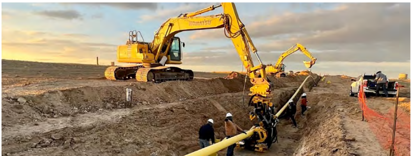
Note: Minimum of two pieces of lifting equipment are required at tie-ins (not including excavator that powers field press) Not seen in photo: Lifting equipment behind camera.
